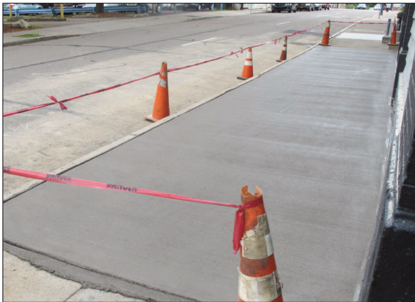
The new sidewalk recently installed where stairs used to be located along West Second Street between Washington and Cherry streets. The stairs were removed because they were in disrepair and were considered a safety hazard.
